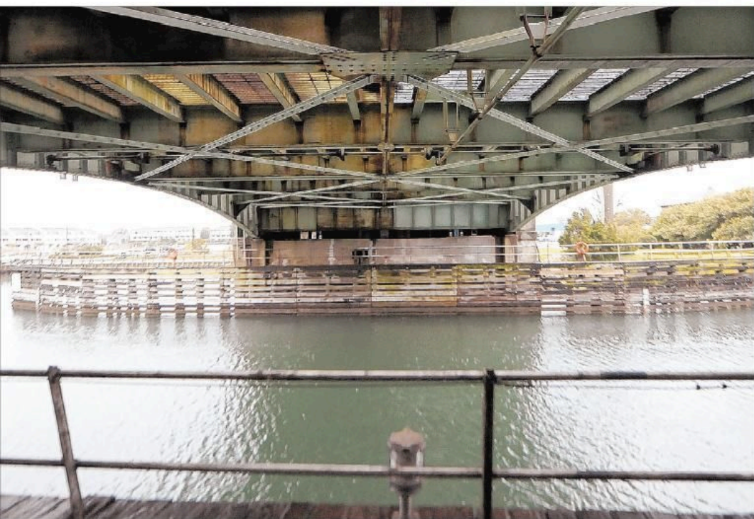
The Wrightsville Beach drawbridge is lifted with a mechanism called the Hopkins drive system, which is among the last of its kind in the state of North Carolina. Photos by Paul Stephen
